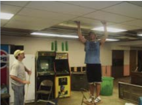
Above: Two of the mission team are shown renewing the ceiling in the church basement.
